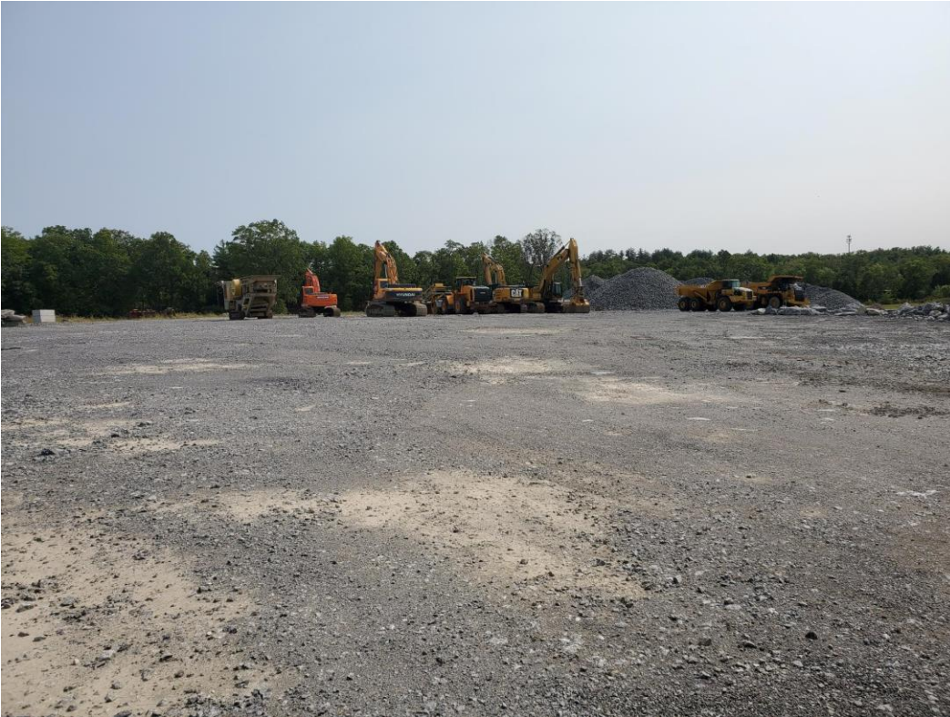
Site with equipment
