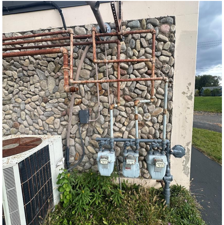
3 Gas Meters & 4 Electric Meters
